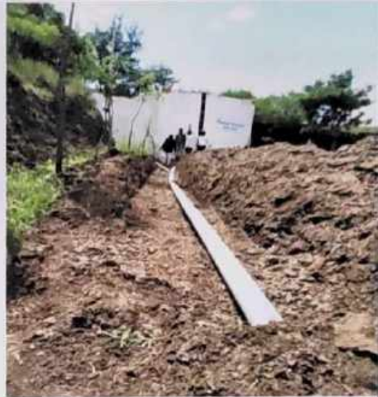
Outlet tank to bore- well
