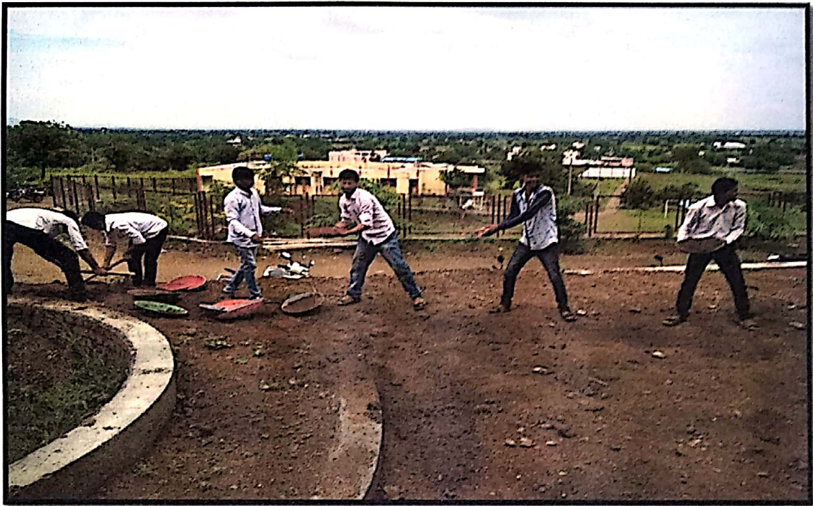
A horizontal wall was constructed on the slope in front of the main building of the college. Students at work
