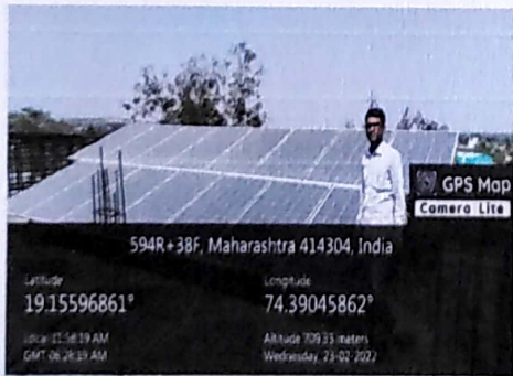
Solar project Ladies Hostel 5KW
