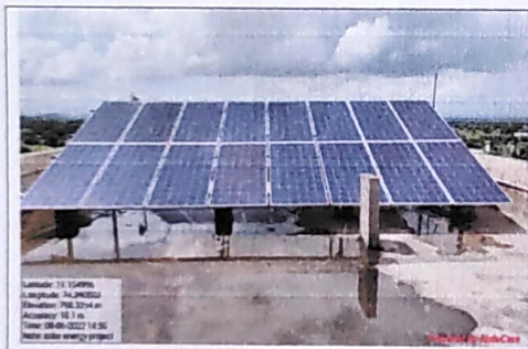
Solar Project Main Building 10KW
