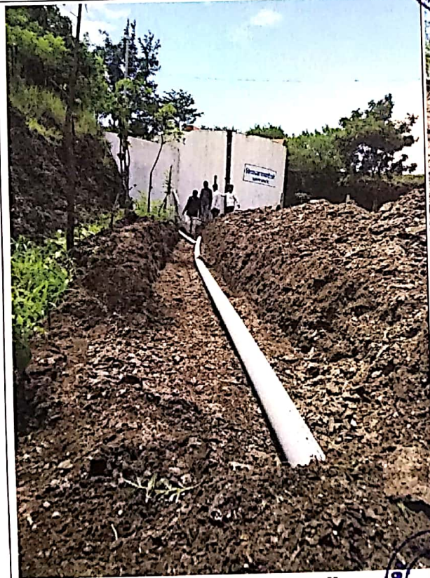
Outlet tank to bore- well
