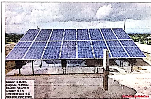
Solar Project Main Building 10KW
